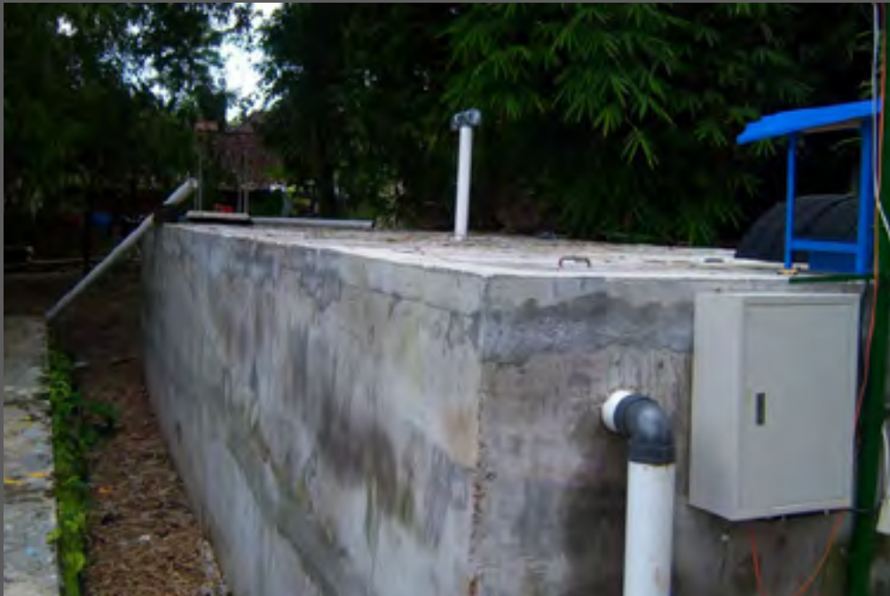
Septic tank vermibiofilter
